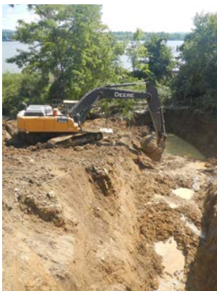
Title: 08-29-16 MP 3.01 unapproved ground disturbance in wetland A14-SPLR- W100 at Hudson River HDD west.
