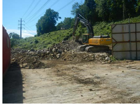
Title: 08-28-16 MP 3.00 upland coffer for spoil storage constructed at Hudson River HDD west.
