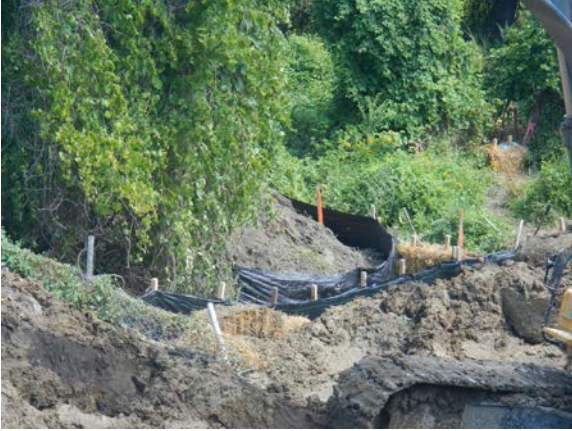
Title: 08-29-16 MP 3.01 unapproved ground disturbance in wetland A14-SPLR- W100 at Hudson River HDD west.
