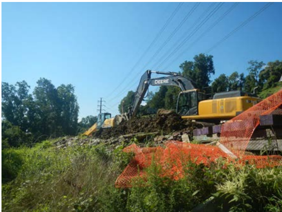
Title: 08-28-16 MP 3.00 upland trench spoil from HDD centerline stored at Hudson River HDD west.
