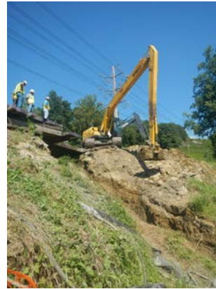
Title: 08-28-16 MP 2.99 excavation over HDD centerline to wetland A14-SPLR- W100 boundary at Hudson River HDD west.
