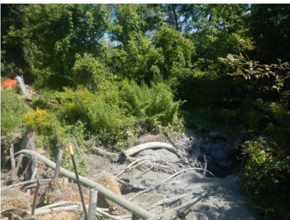
Title: 08-28-16 MP 3.01 submersible mud relay pumps in IR in wetland A14- SPLR-W100 at Hudson River HDD west.
