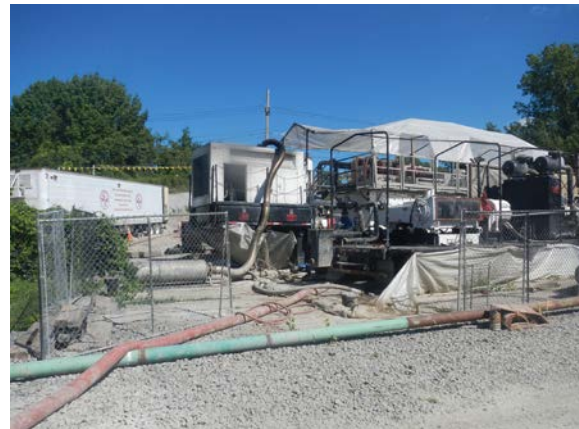
Title: 08-29-16 MP 3.91 mud recycling rig in secondary containment at Hudson River HDD east.
