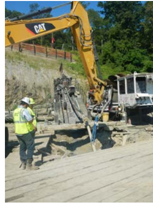
Title: 08-28-16 MP 3.00 deformation in drill stem at rig - Hudson River HDD west during installation.
