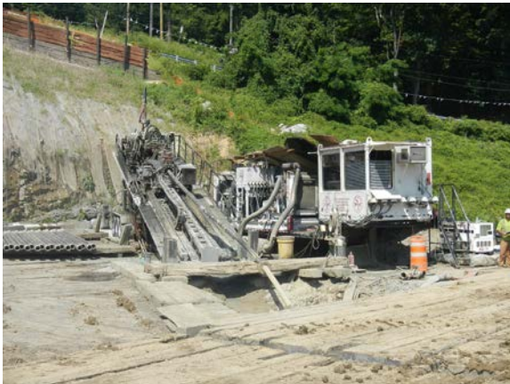
Title: 08-29-16 MP 3.00 deformation in drill stem at rig - Hudson River HDD west during installation.
