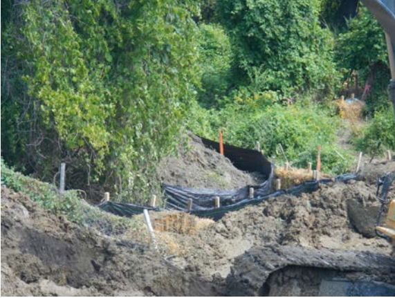
Title: 08-29-16 MP 3.01 unapproved ground disturbance in wetland A14-SPLR- W100 at Hudson River HDD west.
