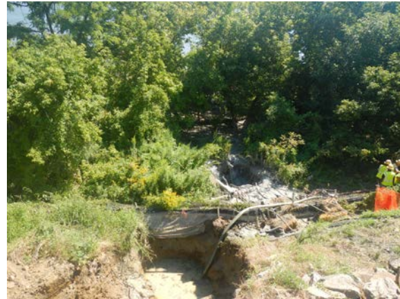
Title: 08-28-16 MP 3.01 submersible mud relay pumps in IR in wetland A14- SPLR-W100 at Hudson River HDD west.
