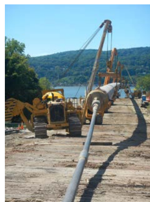
Title: 08-29-16 MP 4.08 pipe segments suspended drill stem at Hudson River HDD east side.
