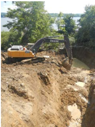
Title: 08-29-16 MP 3.01 unapproved ground disturbance in wetland A14-SPLR- W100 at Hudson River HDD west.
