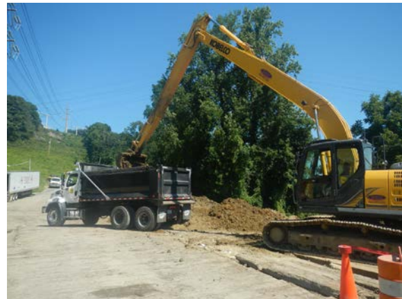
Title: 08-28-16 MP 3.00 upland trench spoil loaded onto dump truck at Hudson River HDD west.
