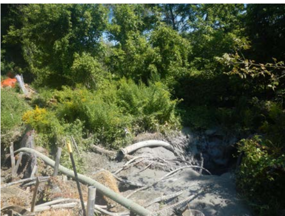
Title: 08-28-16 MP 3.01 submersible mud relay pumps in IR in wetland A14- SPLR-W100 at Hudson River HDD west.
